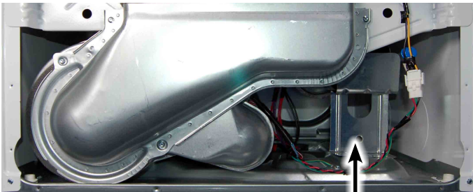
High-Limit Thermostat, Thermal Cutoff, & Heater Area
